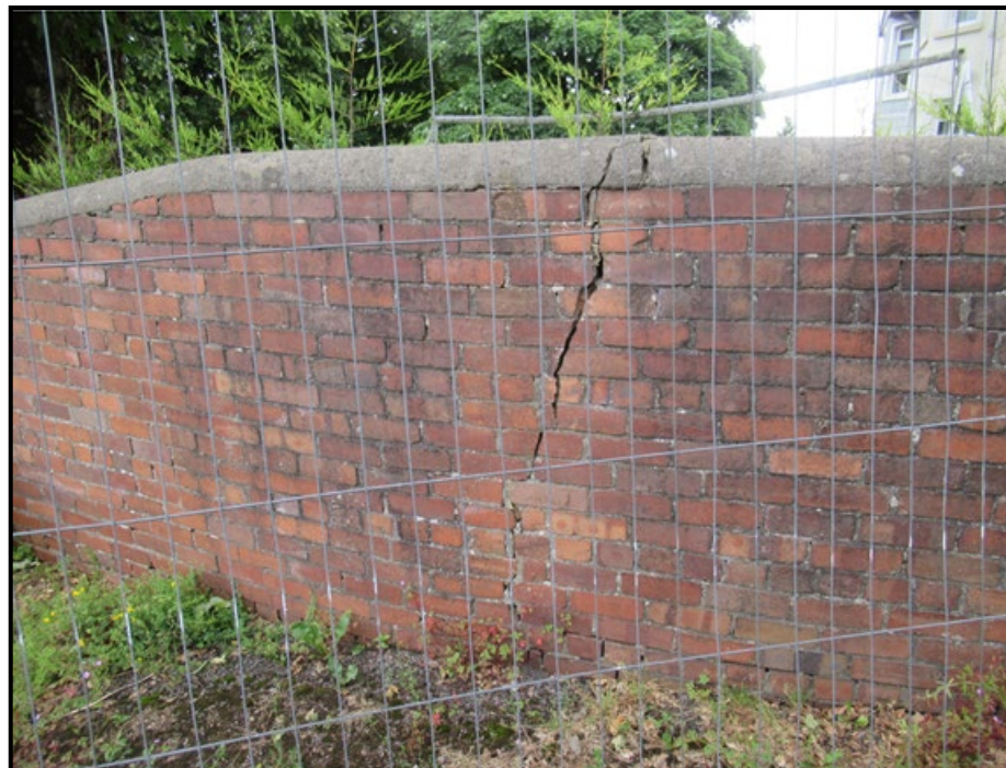
Photograph 2 – Evidence of crack in boundary wall
