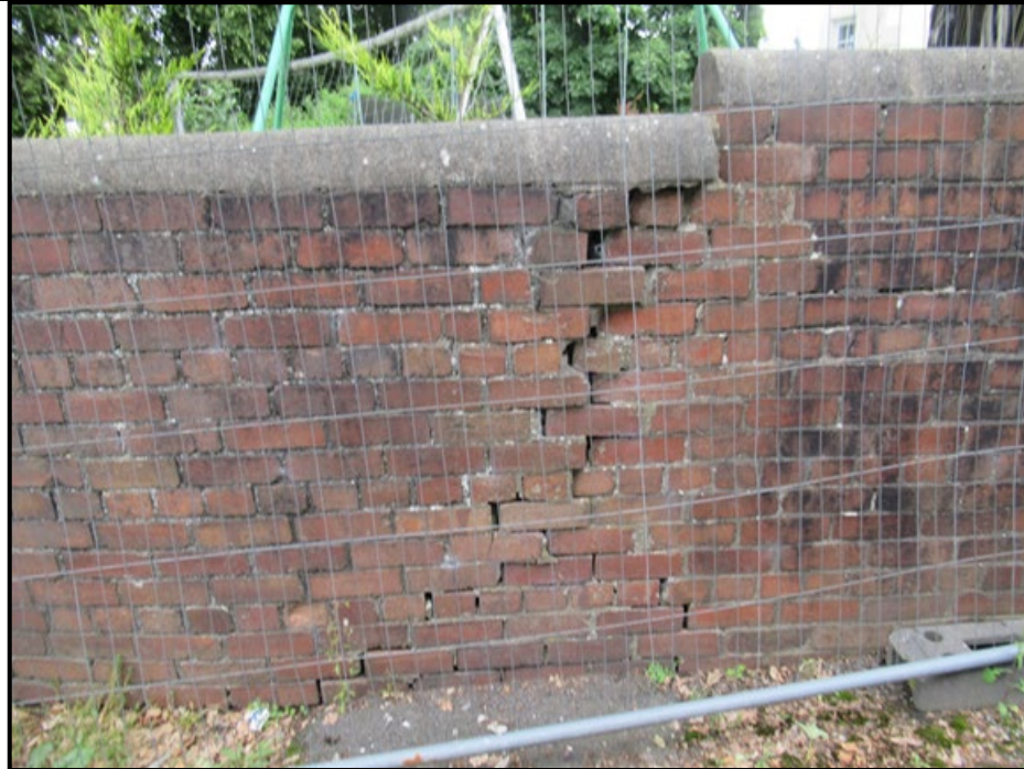
Photograph 3 – Evidence of cracks and movement in boundary wall
